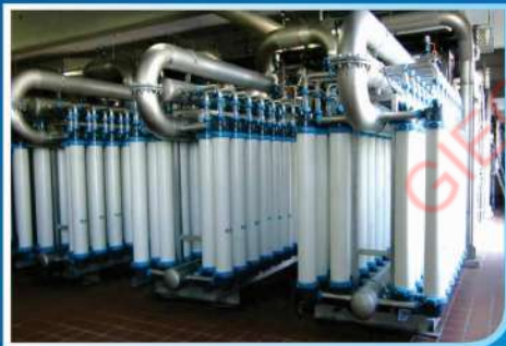
Ultra-Filtration System (UF)
