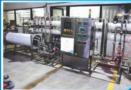
9.5 M3/Hr. Pure Water Generation System Base on Two Pass RO System with EDI - ION PURE
