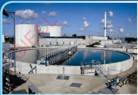
Clarifier for Sea Water & STP & ETP plant
