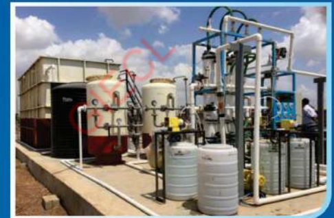
STP Plant 500 KLD
