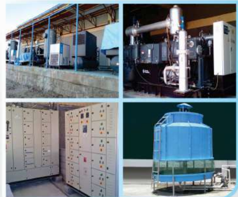
Utilities / Auxiliaries for Bottling Project Such as High- & Low-Pressure Compressor, Chiller, Air Dryer, Filters, Air Receiver Tanks, Cooling Tower, MCCB-LT Panel, APFCR Panel
