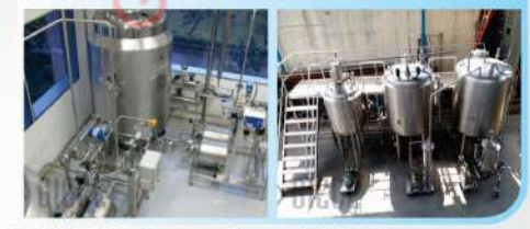
Distribution & Loop System for Pharmaceutical Industries
