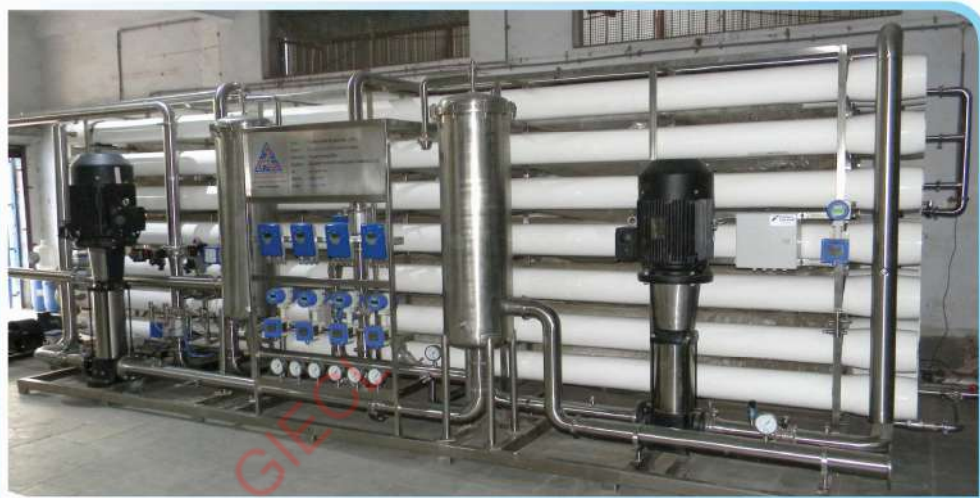
Sea Water Treatment Plant Based on Two Pass RO System with Micron Filter, High Pressure Pump, Digital Flow Meter, Digital TDS & pH meter
