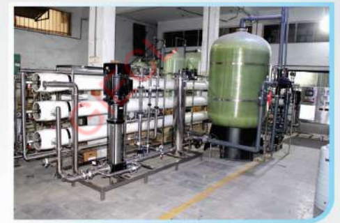
20.0 M3/Hr R.O. System for Boiler, Cooling Tower and Processing
