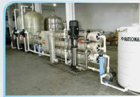
15.0 M3/Hr. RO System with Multi grade filter and activated carbon filter for Township & communities supply
