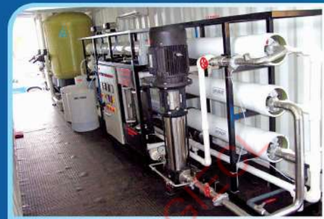
10.0 M3/Hr. Brackish Water Containerize RO System for Civic Supply on Island for drinking and Household application
