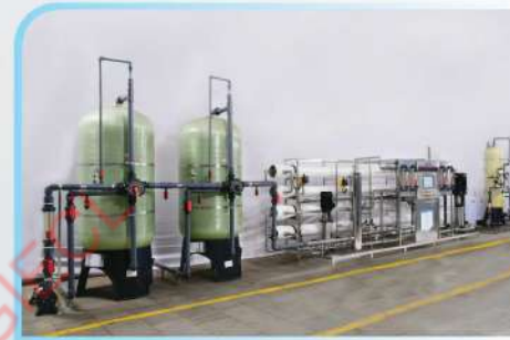
8.0 M3/Hr. Pure Water Generation System Base on Pre-treatment+CSRO+CSRO+MB
