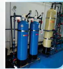
DM Plant + MB Unit + UV + MCF Low Cost Solution
