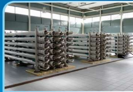
400.0 M3/Hr. Sea Water Desalination R.O. Plant
